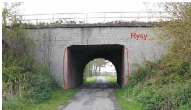
Rys. 5. Wiadukt żelbetowy (pod torem nr 2) [9] Fig. 5. Concrete viaduct (under railway track no. 2) [9]
